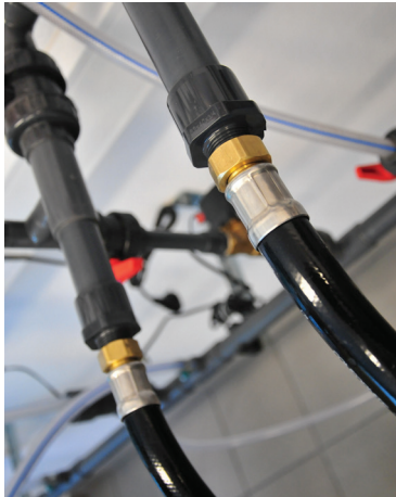
Thread ends: into piping
